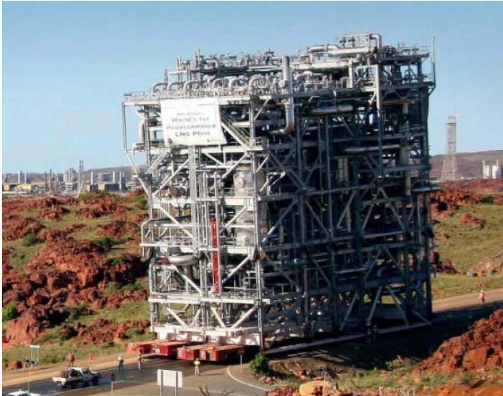
One of the NWS Train 5 (4.4 Mtpa) modules
