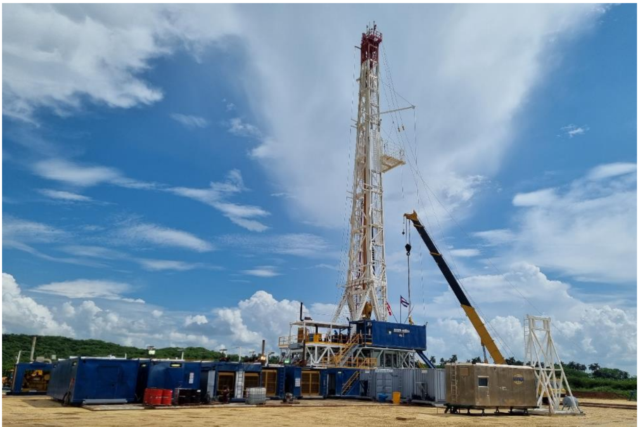
Figure 1 – Derrick of drilling rig raised at the site of the Alameda-1 exploration well
