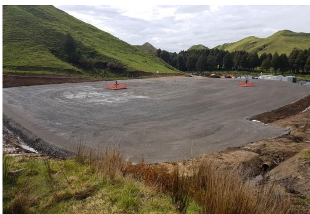
Figure 1 - Completed Pukatea drilling pad with existing Puka-1 and Puka-2 suspended wells protection zones visible
