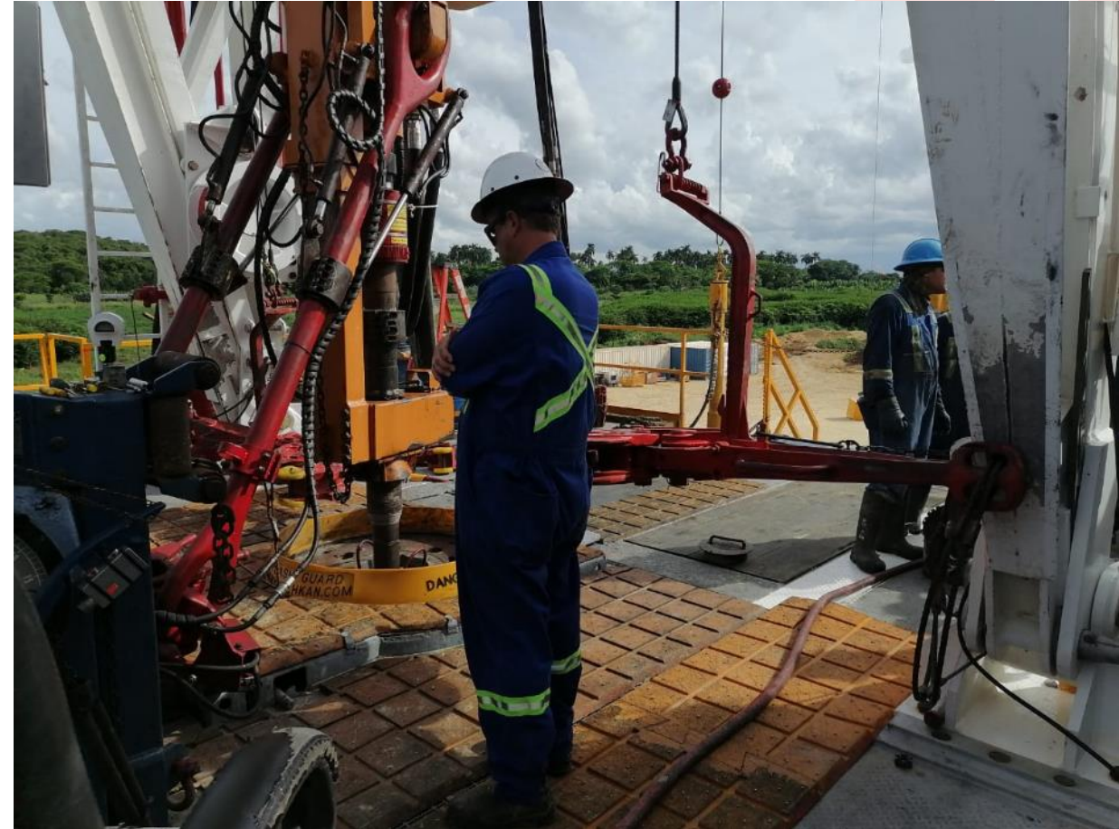
Melbana's Drilling Manager inspecting drilling operations at the Alameda-1 site on 14 September 2021
