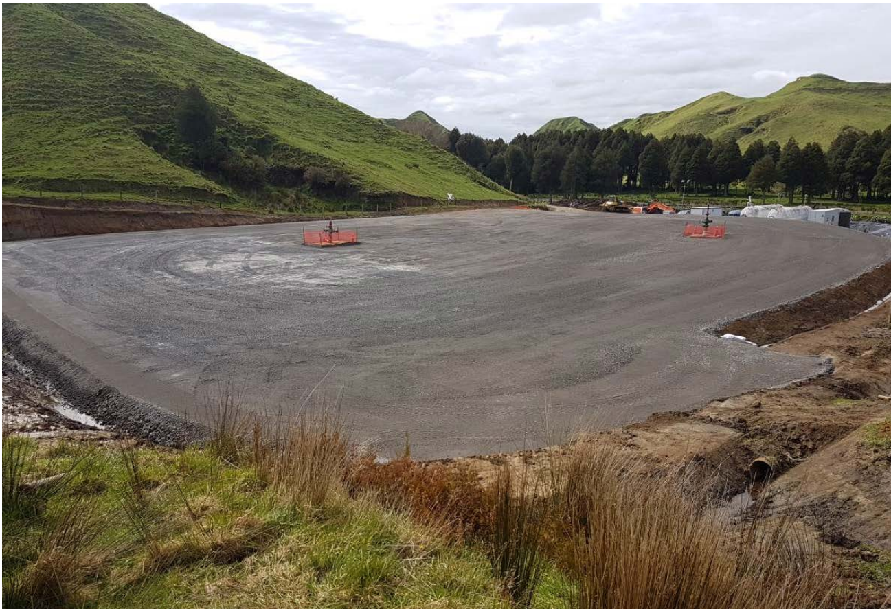
Completed Pukatea drilling pad with existing Puka-1 and Puka-2 suspended wells protection zones visible
