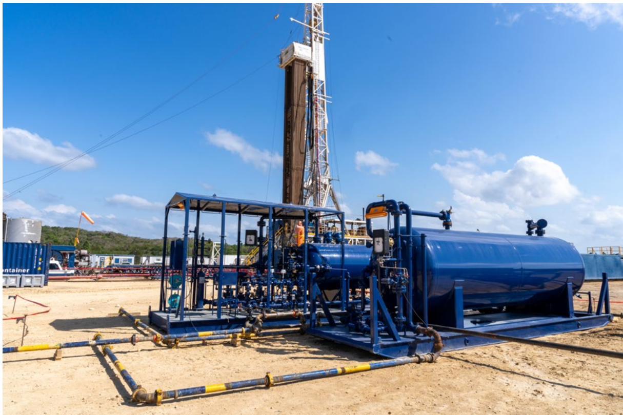
Figure 3 - High pressure test separator ready for testing to commence
